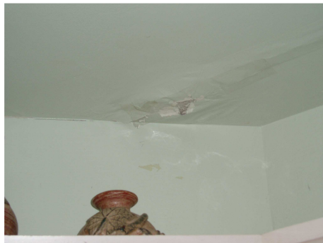
Kitchen Ceiling Crack
